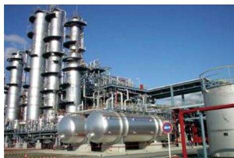
Figure 1. Vinyl chloride monomer plant.
